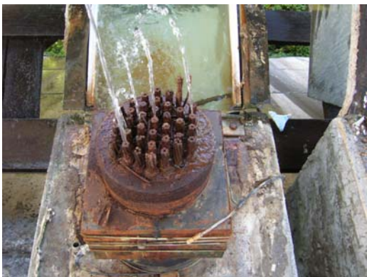
Figure 8 – Typical Corroded Anchor in 2008 (Note Water Spraying Out of Strands)
